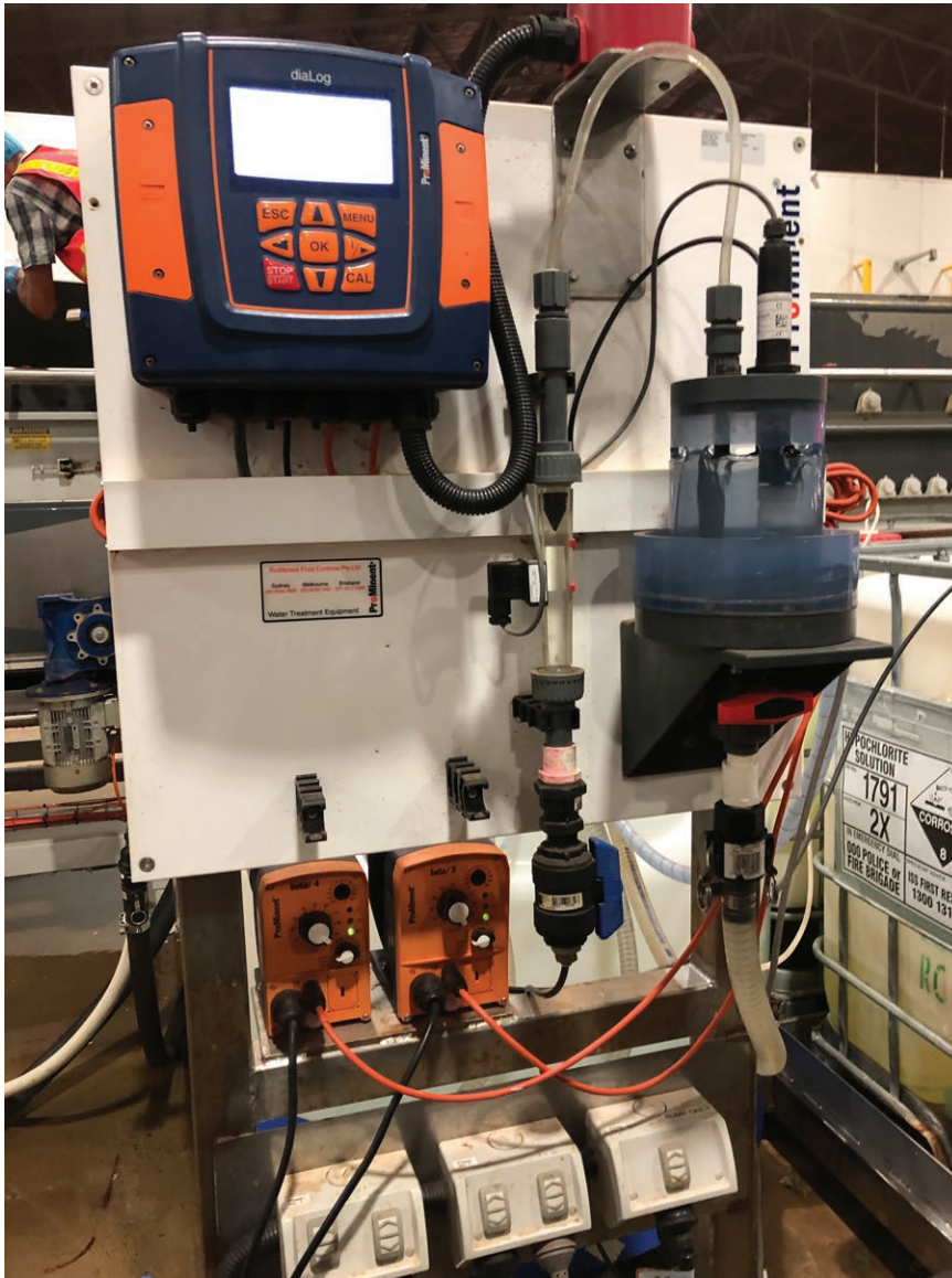
Figure 35. An automated chlorine injection and monitoring system.
