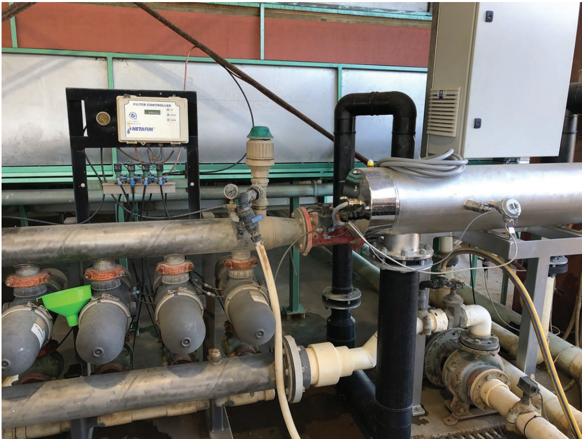
Figure 25. Wash water filtration.
